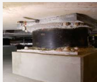
High damping rubber bearing under the building.
