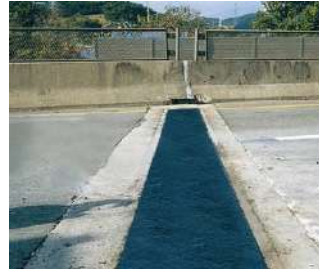
Asphaltic plug joint used in connection of bridges
