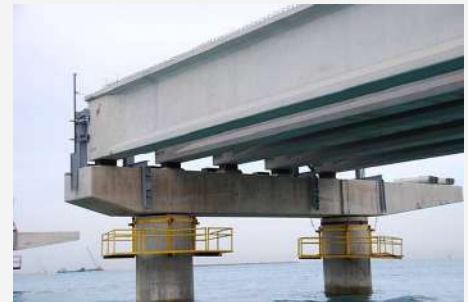
Round PTFE laminated bearing pads on skew bridge.
