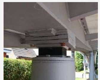
High damping rubber bearing under the flyover.
